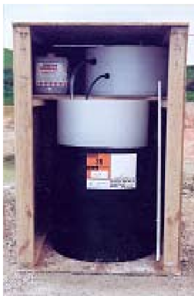
Example of an on-site chemical flocculation system
