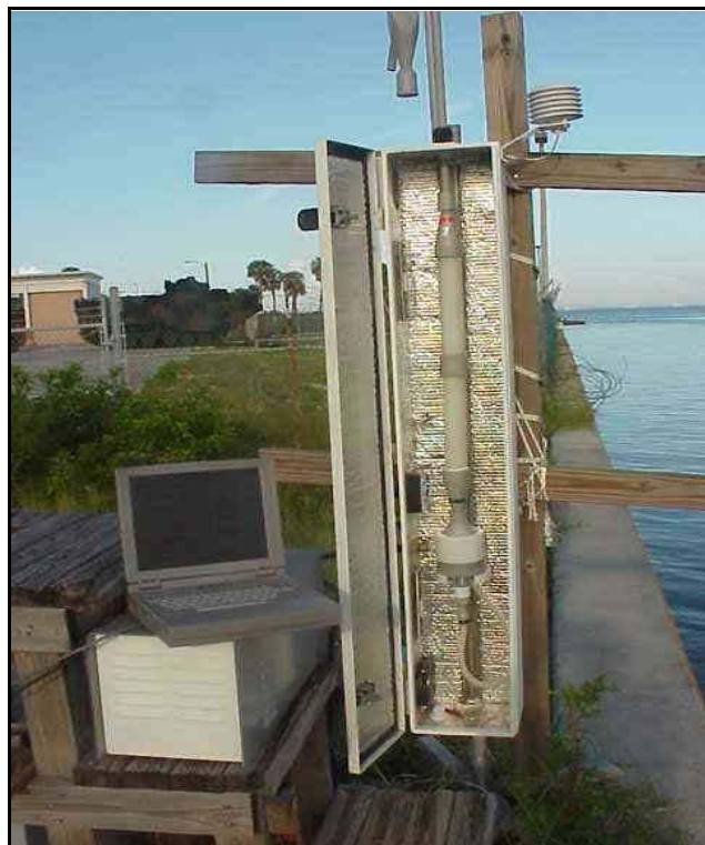
Figure 1. HiC-IOGAPS installed at the seawall near the eastern end of the Gandy Bridge, Tampa, Florida.
